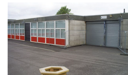
■ Chryston Primary School, Glasgow CLASP System built school with failing concrete Cladding panels
