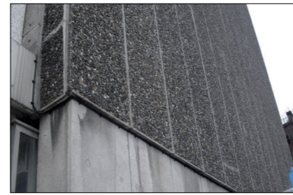
■ Typical 1970's office block before refurbishment With failing concrete panel cladding.
