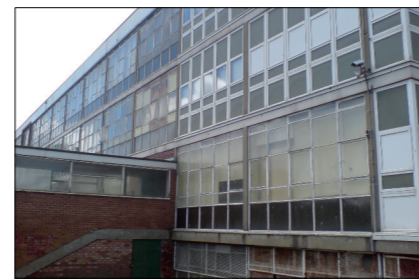
■ Typical system built school before refurbishment with large areas of inefficient glazing and cladding.
