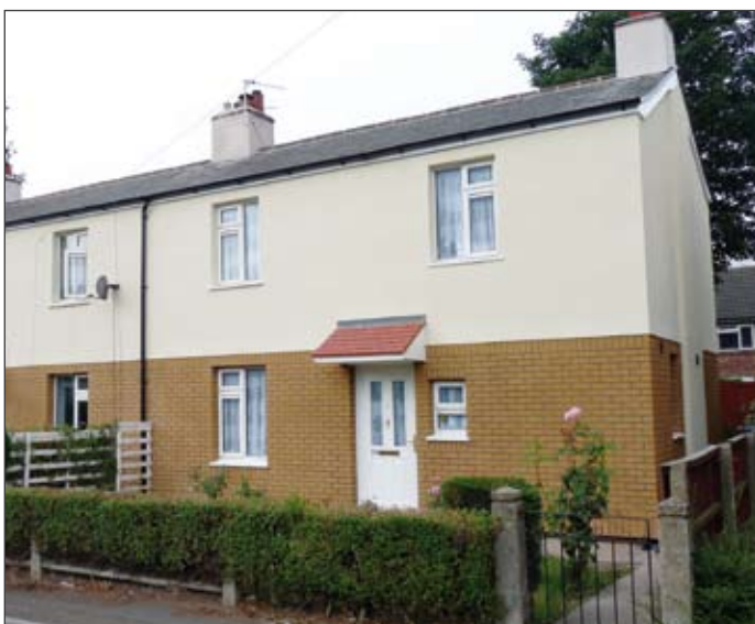
Residential Refurbishment Project: High Build EWI System with Brick Effect Finish to Ground Floor & Acrylic Finish to First Floor
