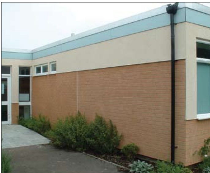
School Refurbishment Project: Heavy Duty EWI System with Brick Effect & Acrylic Finishes
